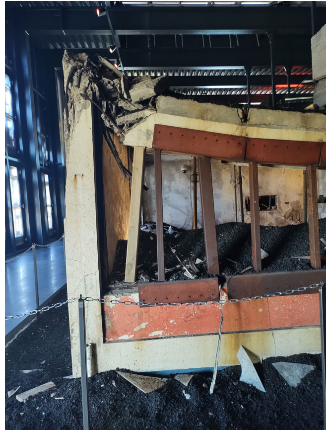
Figure 16: Gerðisbraut 10 forms the central exhibit in the Eldheimar museum on the island of Heimaey. Visitors cannot enter the house due to the structural damage caused by burial by several meters of volcanic ash, however interactive technology allows remote viewing of individual rooms. Photograph: Rh. H. Meara.
