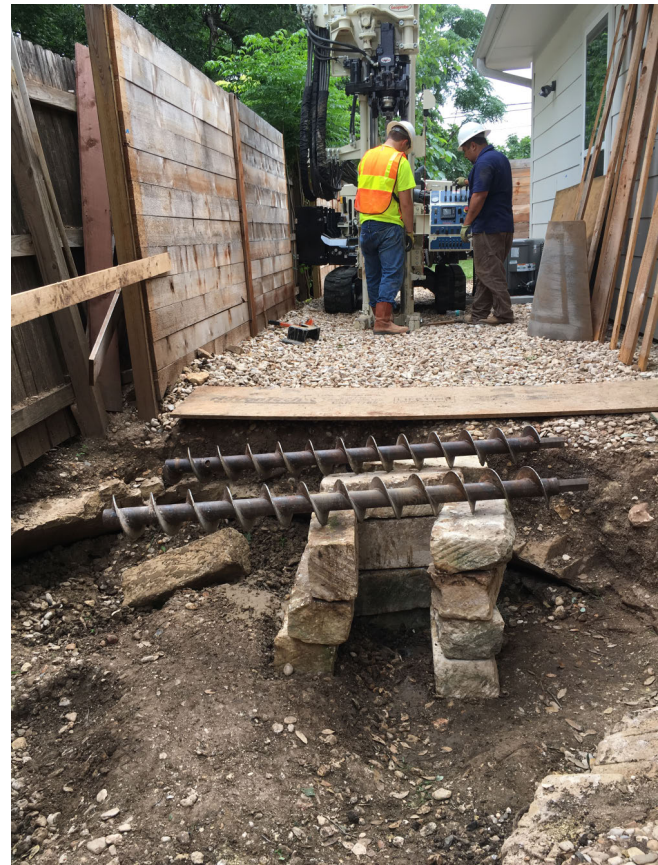
Figure 15: Picture showing the location of the cistern (old water well) and drilling at borehole location B-1. Resistivity profile P8 was surveyed along the corridor between the wooden fence and the house.
